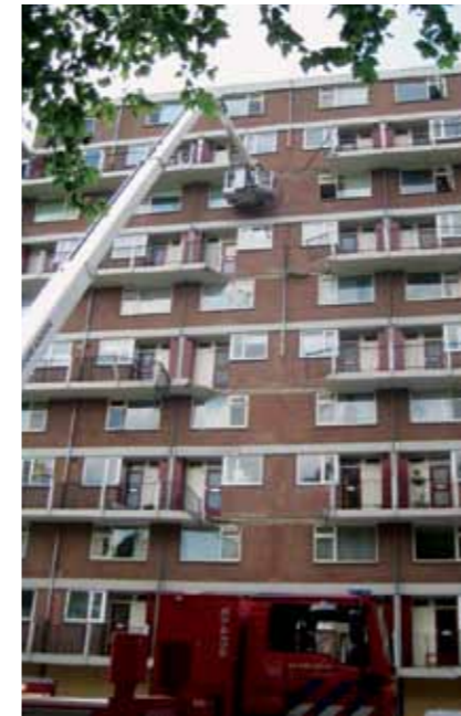
Overview after the fall of the gallery slab on the 5 th floor.
