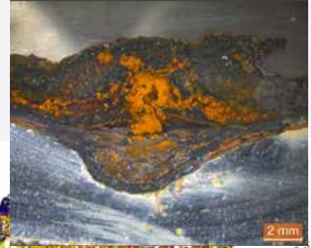
Microscopy of Pitting Corrosion in steel pipe
